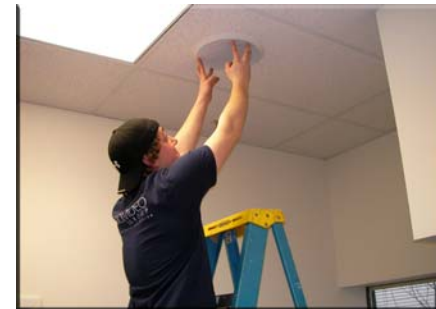
AVG at Work: T.J. checks out a ceiling speaker. We pride ourselves on being reliable and responsive to our church's needs.
